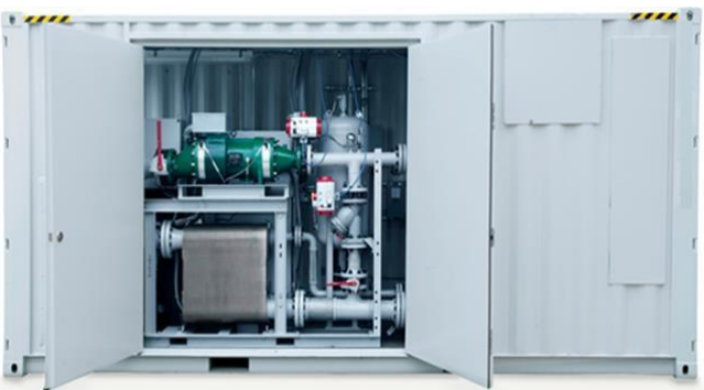
Figure 4. Inside of Containerized ORC System
